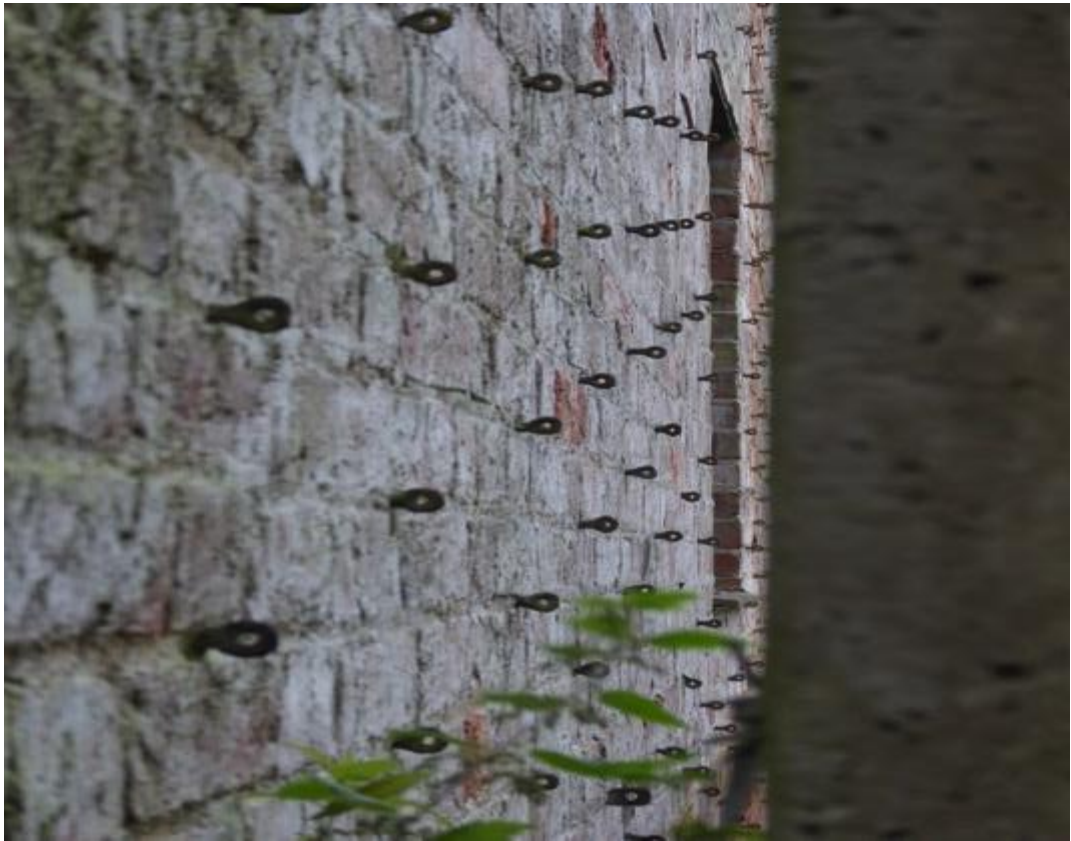
Glimpse of WKG North wall also showing nails for plant support wiring.
