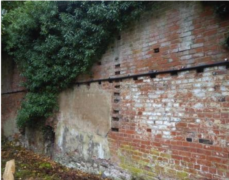
North wall of Frameyard seen from the North Showing plaster & holes for lean-to buildings
