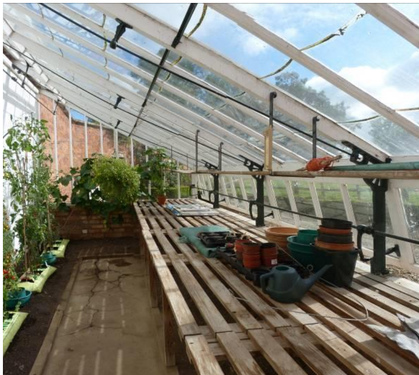
Interior of Messenger greenhouse showing parts of the original ventilation system
