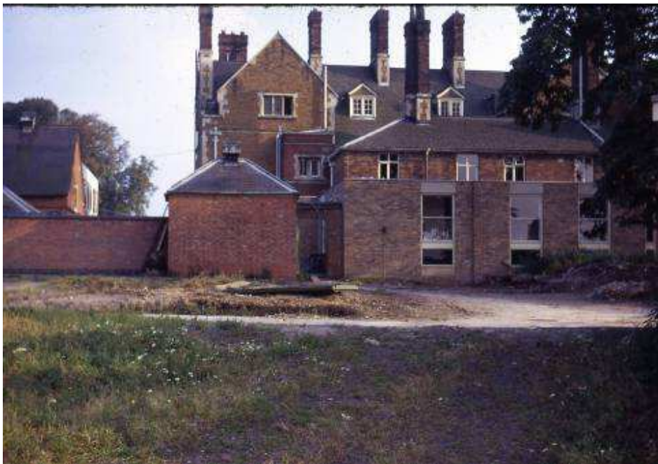
The Walled Garden partially demolished in 1975. The remaining greenhouse can still be seen in the upper image and the square building is the apple store.
