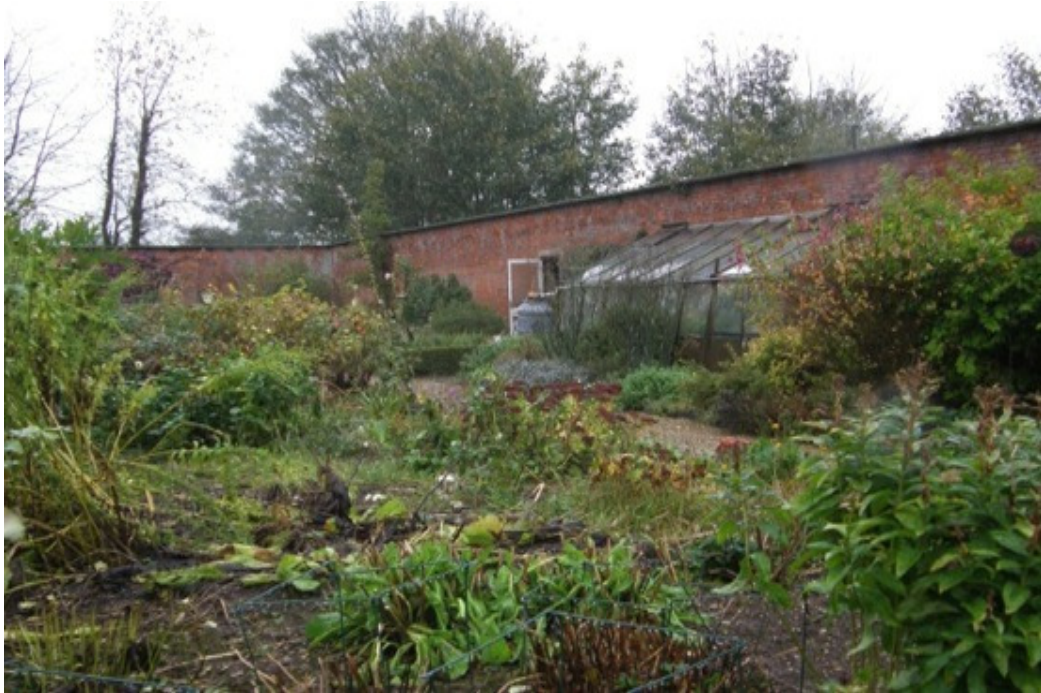
The NE and NW walls meeting in the Northernmost corner. A modern lean-to glasshouse is shown and the door into the backshed housing the pigswill oven
