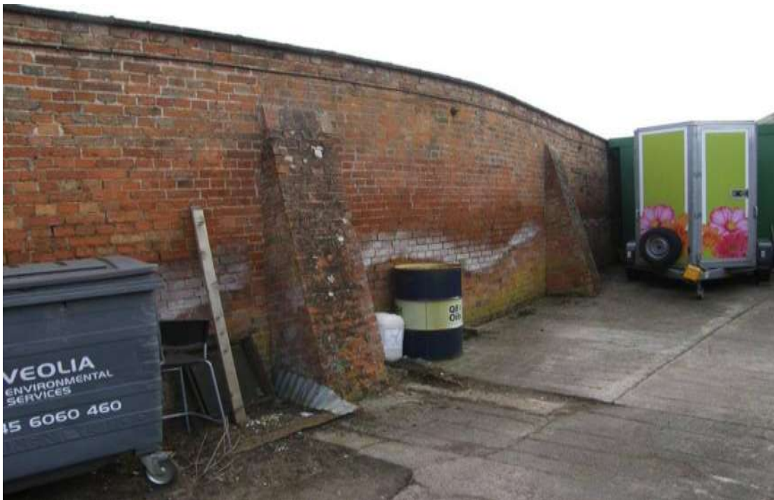
The curved North all from the outside of the WKG showing the buttresses
