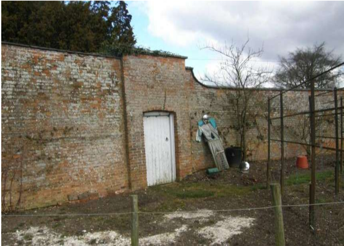
The disused door in the North East side of the WKG showing the difference in height between the curved North wall and the straight side wall
