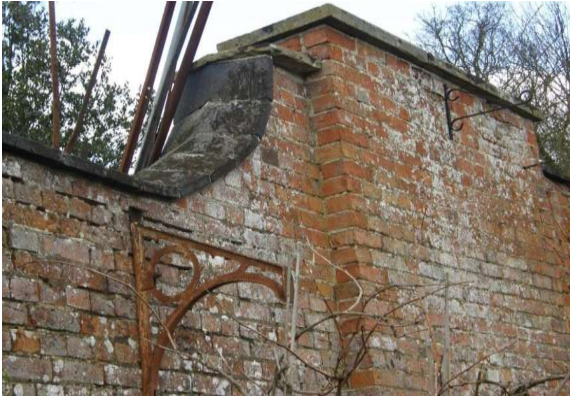
The wall bracket in the foreground is one of a series equally spaced along the West wall and the western side of the North wall. These were used to support a shelter for the plants from the intense heat of the morning sun after a frosty night
