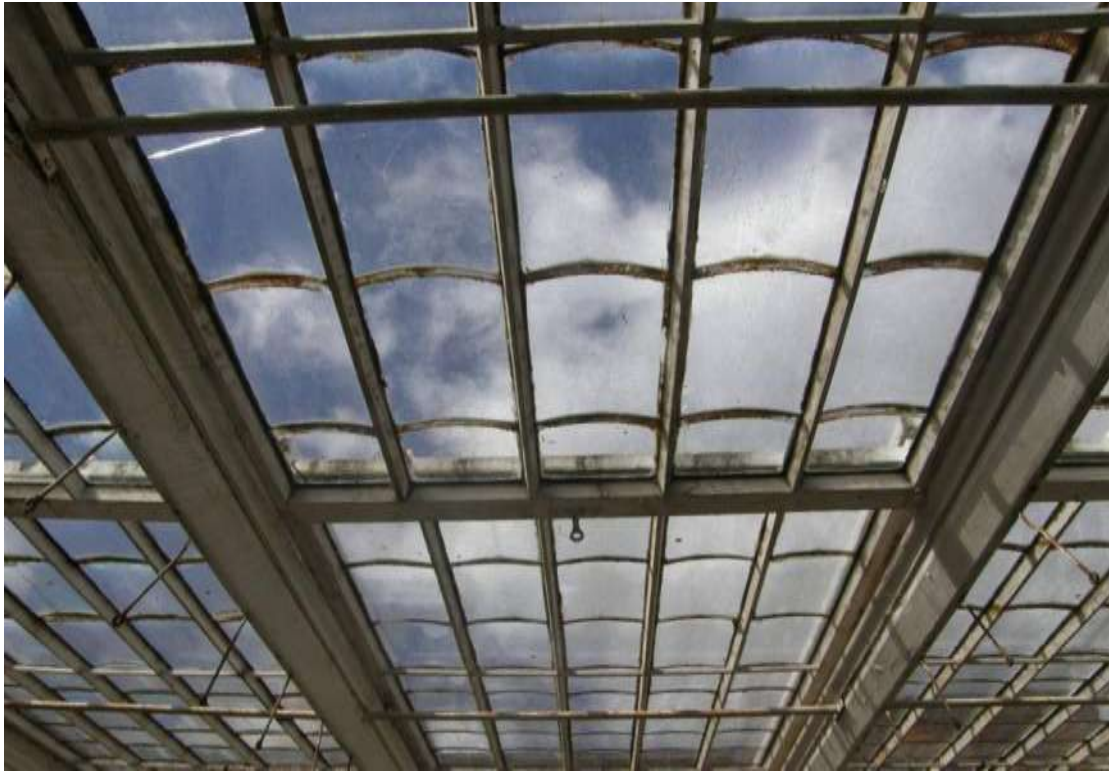
The roof of the vinery showing the lower edges of each pane of glass designed to provide better drainage
